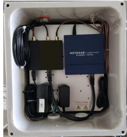
Example of installation with communications equipment
